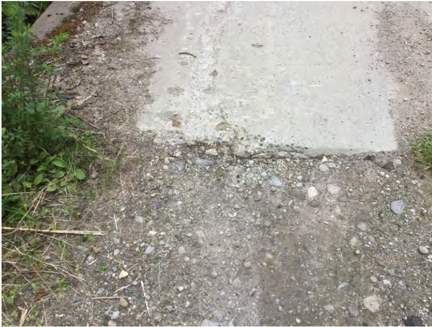
Damage to left bank slabs
